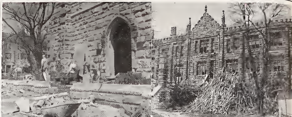
SEWANEE CONSTRUCTION CONTINUES as army of workers toil simultaneously on expansion of chapel, renovation of Walsh Hall, and the construction of a new wing of Emerald-Hodgson Hospital.
