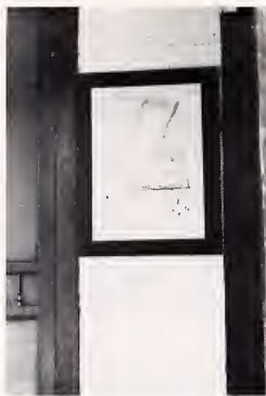
Local art on one porch. Unremovable except by demolition. Fortunately it is in the best of taste and artistic style (vandal, circa 1950's) and not obscene.
