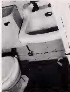
All bathrooms are so small that the photographer could only hold his camera in the door and shoot. The stall shower is as close to the toilet as the sink.
