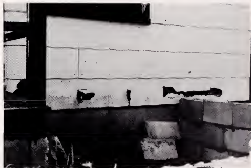
Not only are the walls uninsulated, but many of the shingles are broken, allowing the wind to literally blow right through. Windows fit within their frames with gaps of up to an inch, creating high heat bills and bug populations.
