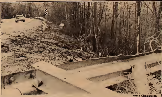
Highway 64, west toward Cowan on Sewanee Mountain, poses numerous problems for drivers and engineers alike. Shown above is the scene of an accident involving a tractor trailer, not far from the landslide for which the state has contracted a firm to repair. See page 12 for details.
