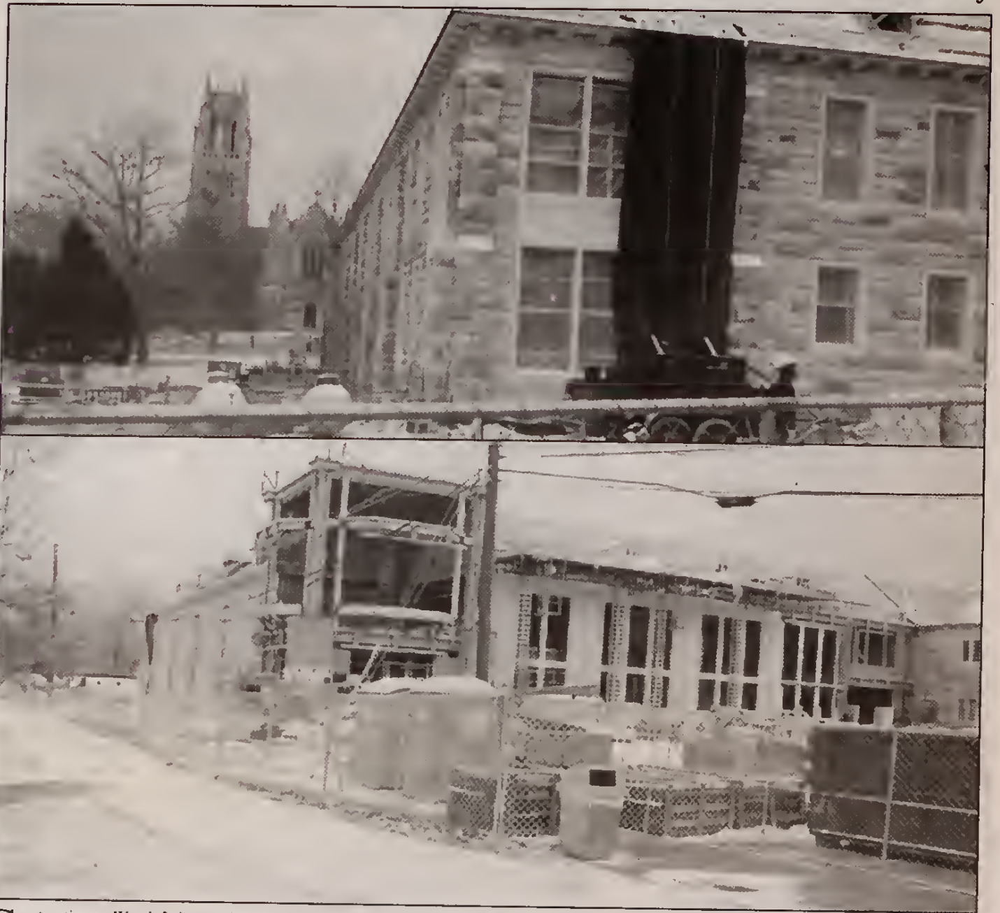
Construction on Woods Lab was visible as snow fell on the campus on Wednesday. "The Spencer Hall addition to Woods Lab is on budget and on schedule for completion in late summer or early fall," says Director of PPS Marvin Pate.
