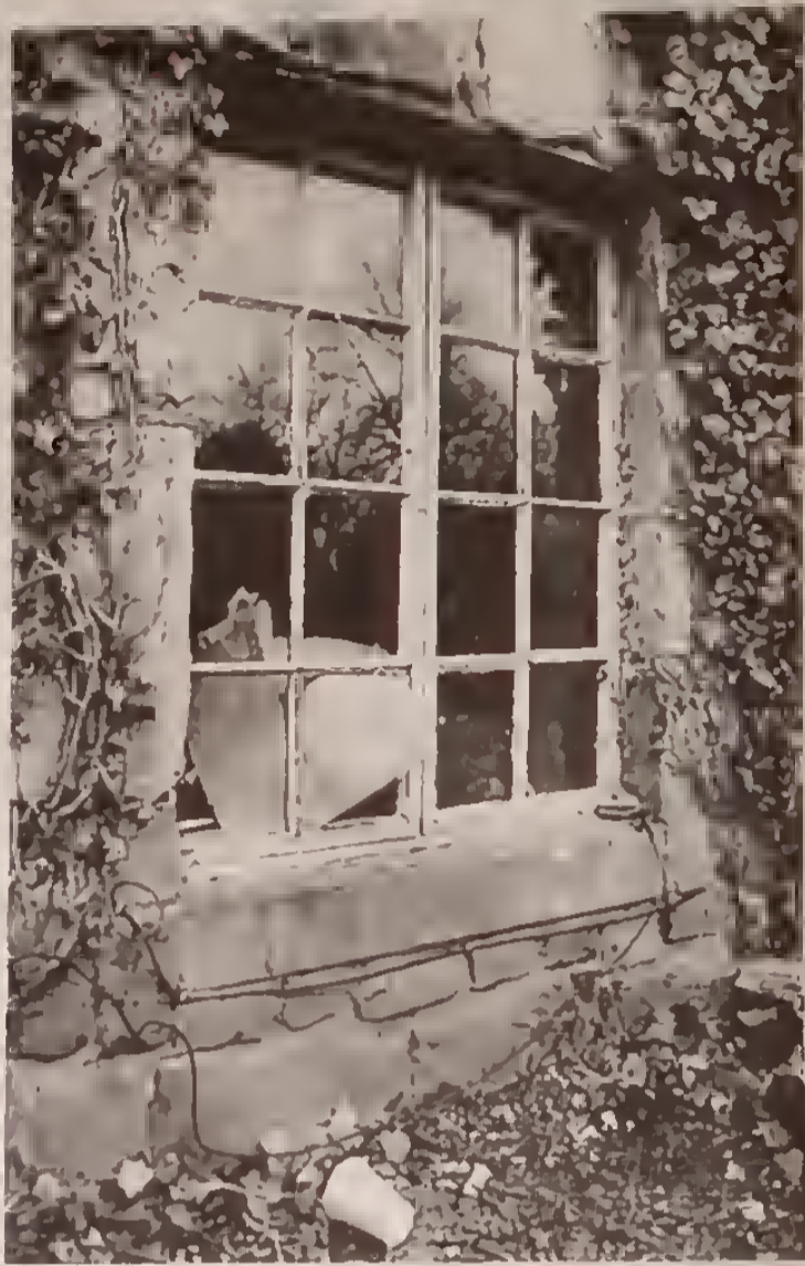
Broken windows are a common sight at several of Sewanee's fraternity houses.
