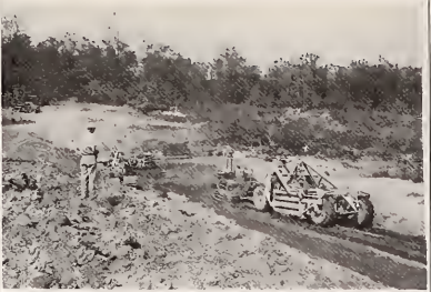
NEW DAM —Work is nearing completion on the earth-packed dam which will create a 15.6 acre lake approximately one mile east of the library. The dam is 529 feet long, 28 feet high, and will contain 13,412 cubic yards of dirt and clay. It will cost about $5,000.
