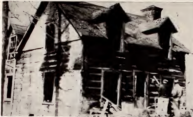
Two workmen survey the blackened ruins of the Thomas P. Govan home which was gutted by a disastrous fire last Thursday night. Dr. and Mrs. Govan, like many of the firmers, were watching a movie when the alarm was given, and the blaze had reached an advanced stage before the Fire Department arrived. —Purple Photo by Keiser-Conner Studio
