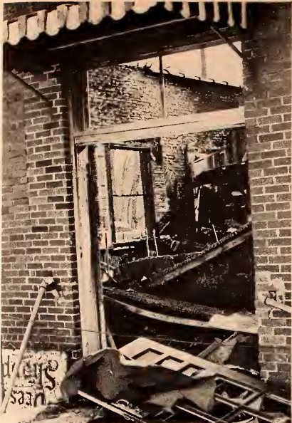
Fire totally destroyed the Village Dress Shoppe Monday, March 31. The blaze, which started about 5 p.m., was finally extinguished at 1 a.m. Fortunately, the firemen, with the aid of their new equipment, were able to prevent the fire from spreading to the other half of the building. However, several of the fire fighters suffered from smoke inhalation, and one was hospitalized.
